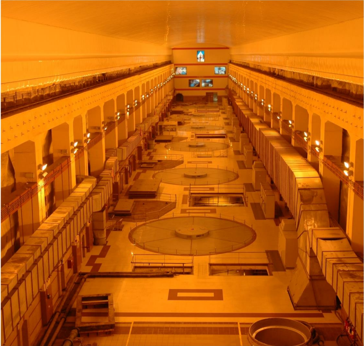
Power House of 1500 MW Nathpa Jhakri Hydro Power Station, Jhakri (HP)
